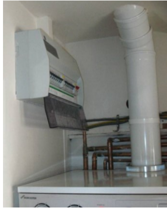
Fuse box up high
